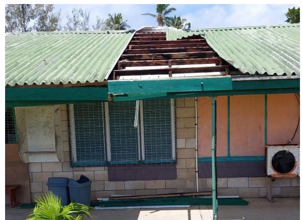
Onesua College - Roof Damage on Computer Lab
