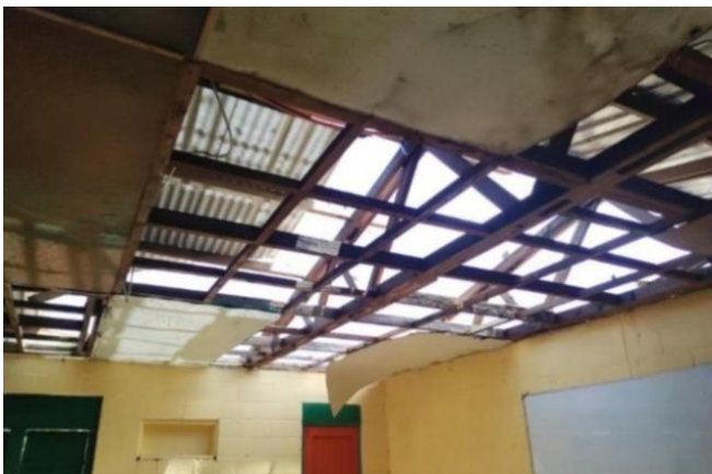
Onesua College – Damage to Junior Science Lab
