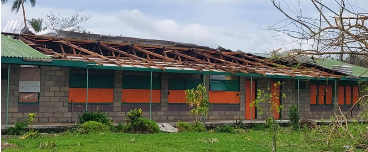
Onesua College Classroom roof destroyed by Cyclone Kevin in March
